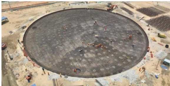
Crude Oil Import Terminal Project, Odisha Blended Cement in Deep Tranche Concrete piles
